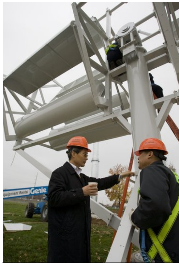
Shane Keyser Seungbae Lee (left), CEO of AeroNet, talked over preparations to install the AES Windjet 5 turbine outside A.L. Huber headquarters in Overland Park recently.
